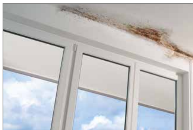
Figure 6: Photograph showing mould growth on the ceiling of a concrete slab adjacent to an exposed slab edge thermal bridge. Condensation forms here frequently as a result of colder interior surface temperatures.
